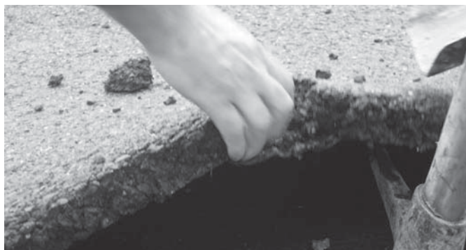
Fig. 1. An extreme example: because of the net usage there is no cohesion between the layers
