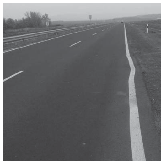
Fig. 2. Because of the build in tissue net, the abrasion layer slipped and a rut has appeared (route 21.)
